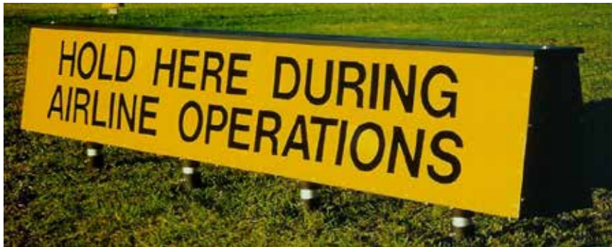
Lighted information sign - installed at Branson, MO.
