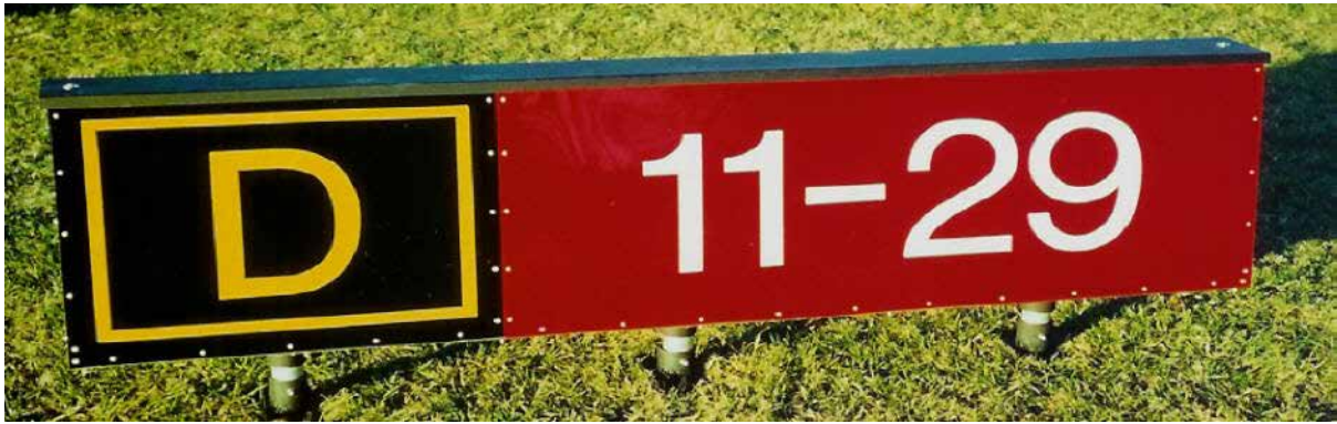
Taxiway Delta, "hold short" runway 11-29 lighted sign.
