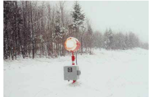
Striplin REIL unit operating in sub-zero conditions in Rockwood, Maine.
